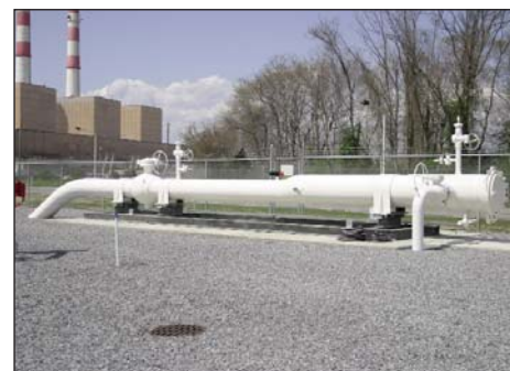
Pig launcher at Iroquois' Northport, NY facility
